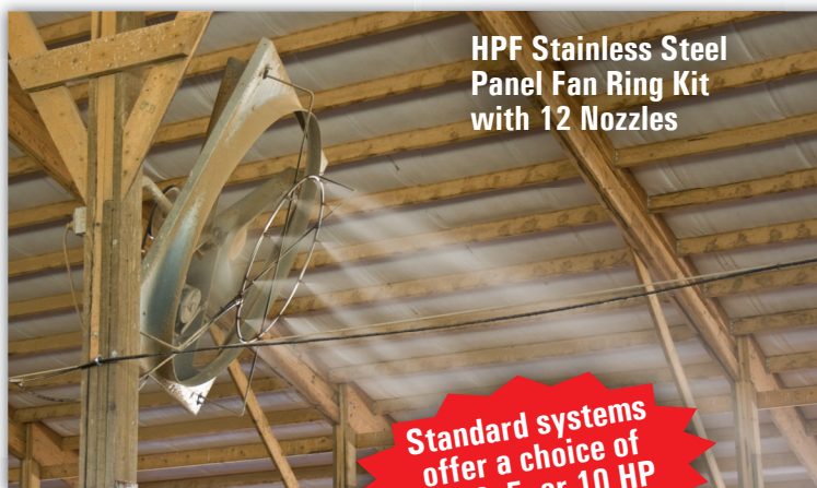
HPF Stainless Steel Lines with 12", 18", 24", or 48" Nozzle Spacing in cross tunnel ventilated barn
